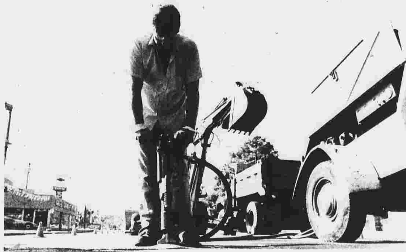
Peter Finks cuts out a temporary patch on an old pothole on Main Street so that it can be refilled. Finks and other town public works employees are busy reading streets for the upcoming winter season.
